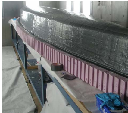
Figure 9: Mold on Levelled Tables
